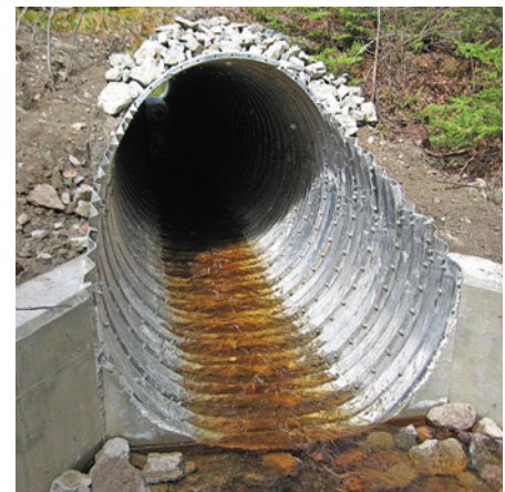
TUNNEL LINER PLATE'S LIGHT WEIGHT MADE IT EASY TO HAND-CARRY SECTIONS TO THIS RESTRICTED ACCESS LOCATION IN TERRA NOVA NATIONAL PARK
